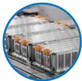
Battery and Energy Storage
